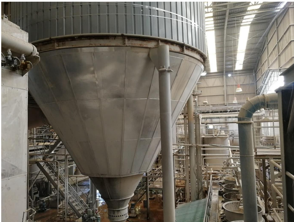
Figure 1.3 - General view of preparation unit
