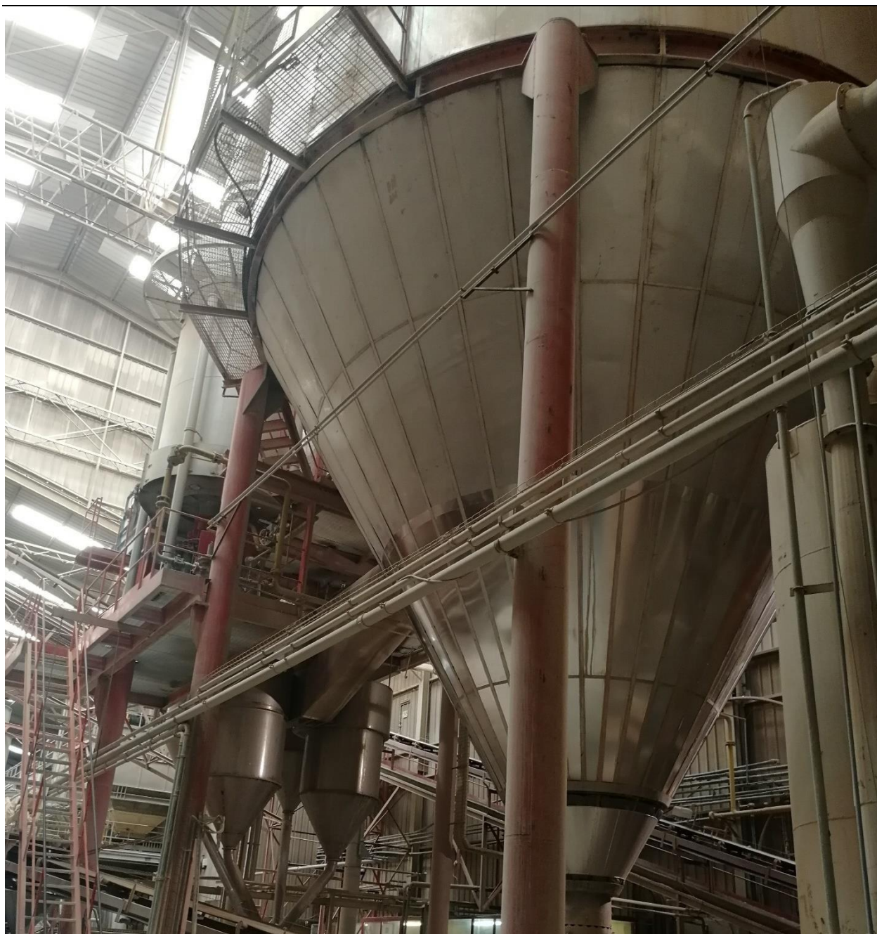
Figure 1.3 - General view of preparation unit
